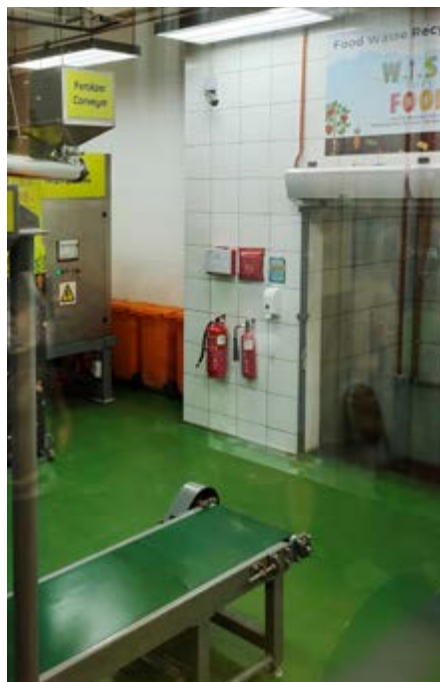
Part of 1 Utama's food waste recycling room which can be viewed by the public
