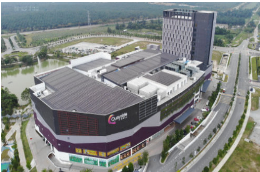
Solar panels installed at Quayside Mall
