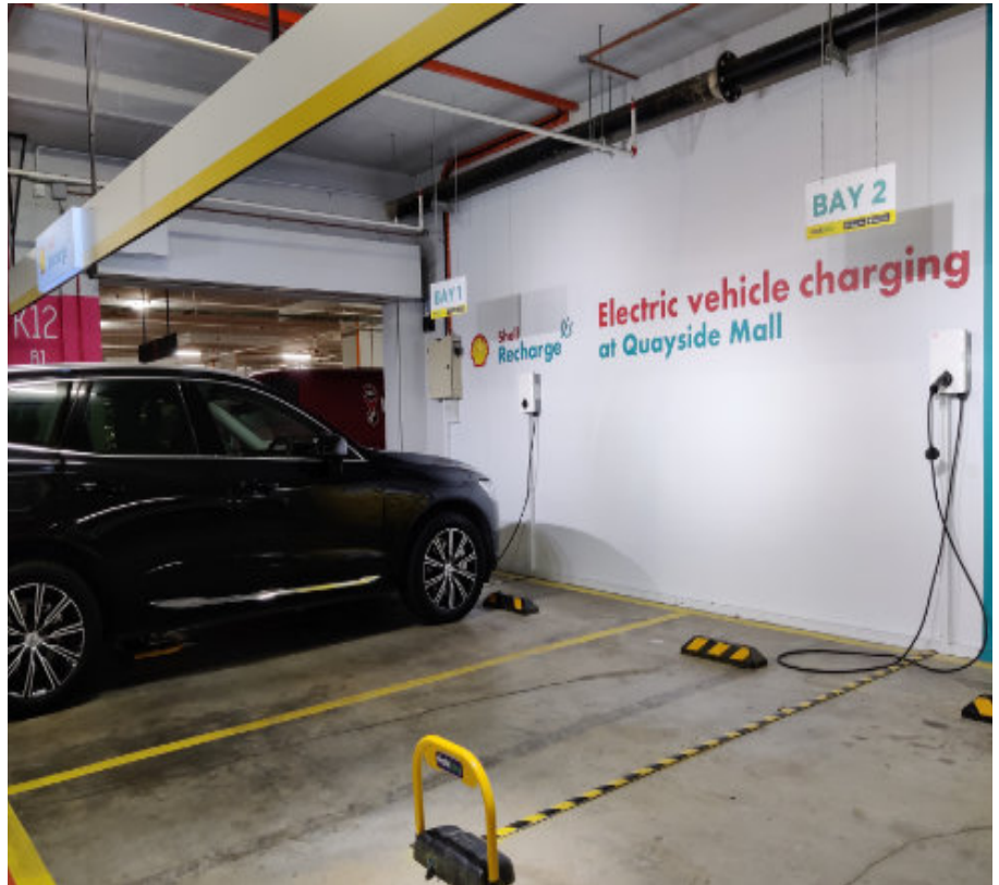
EV charging stations part of its green initiatives
